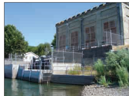
Hydrolox engineered polymer screens have proven to outlast steel screen components in a variety of water-screening applications. Hydrolox screens at the Burbank Pumping Station in Washington.
