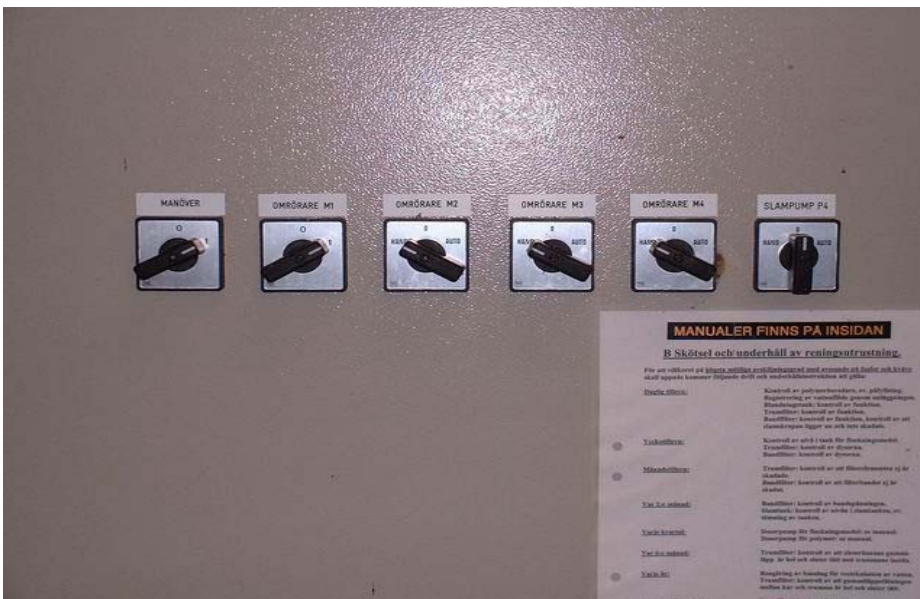
Control panel for mixer tank
