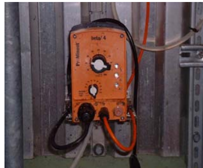
Dosing of aluminium hydroxide.
