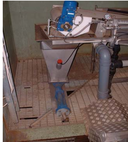
Sludge pump on outlet hopper. "scraper" at the top for sludge removal
